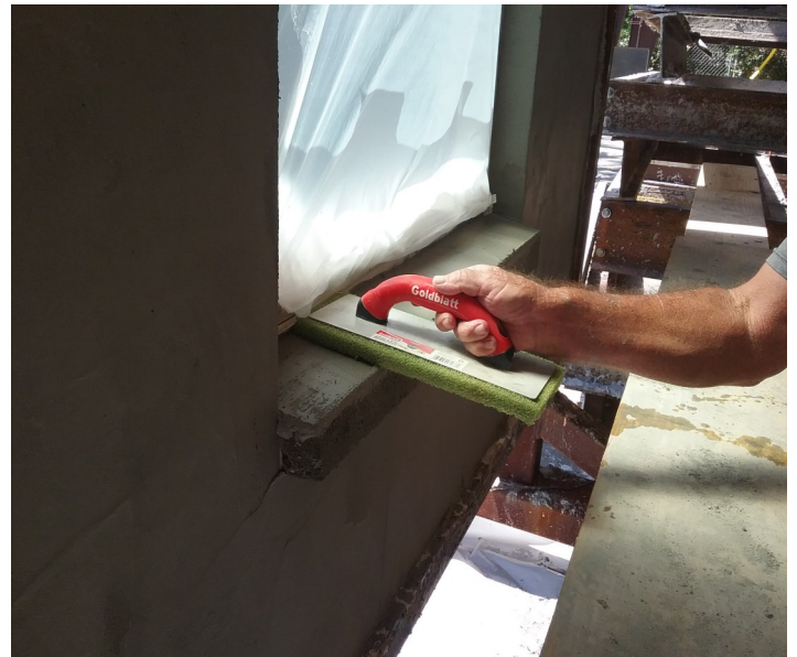
Figure 8-13 Sill is to be Floated. No texture, spray or other impediments to drainage permitted. See Detail 06_06 CMU Sill Slope
