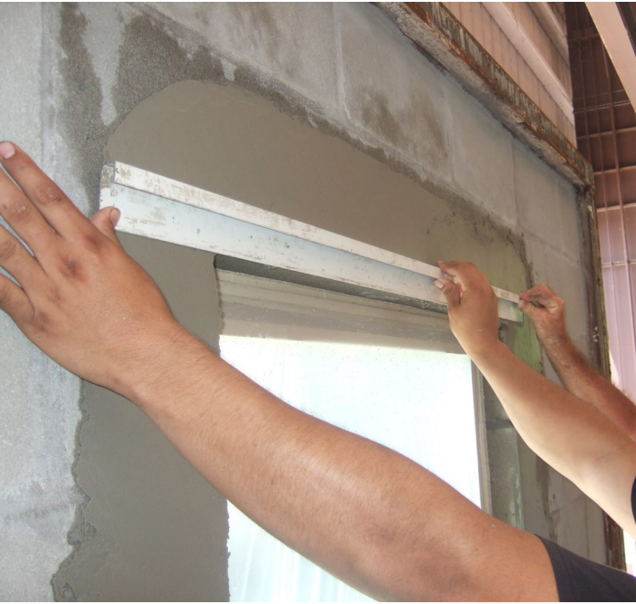
Figure 8-10 Setting a Rod to mud the "arris" (top angle return to the window)
