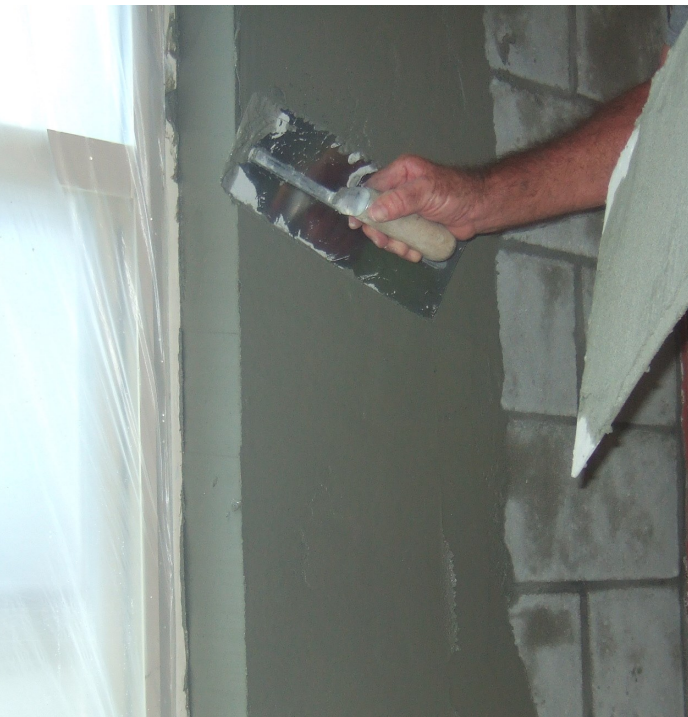
Figure 8-15 Rod "slid off" (upward and outward motion). Trowel removing rod slide-off marks.
