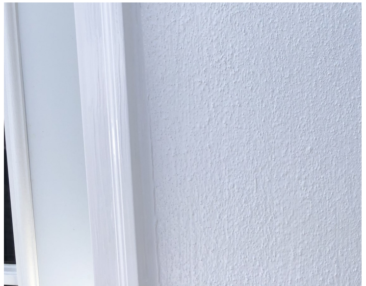
Figure 7-13 Photo of Tooled Sealant Socket after Application of Final Coat of Wall Coating
