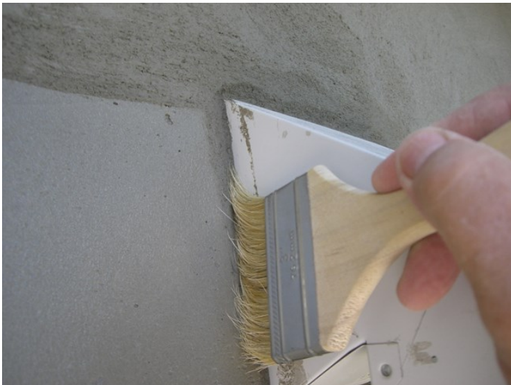
Figure 7-8 After "V" Tooling, the Sealant Socket must be brushed with a brush having dampened bristles. Smooth Edge and Clean Shoulder
