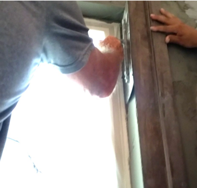
Figure 8-14 Rod set on Jamb Side of the Window Return. Mudding in the return - top to bottom.
