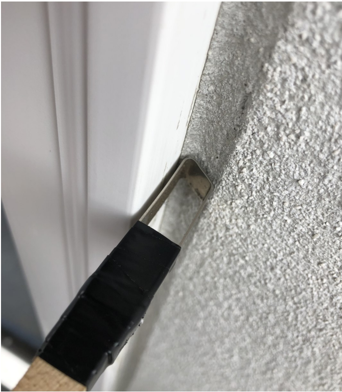
Figure 7-6 Example of Proper "V" Tooling, Brushing, ready for application of Sealant with Spatula
