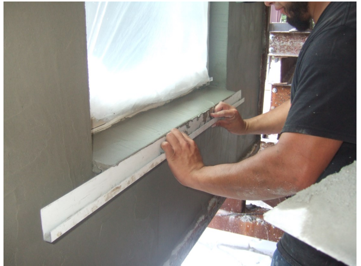
Figure 8-12 Using a Rod to mud the sill to the required slope. (See Detail 06_06)
