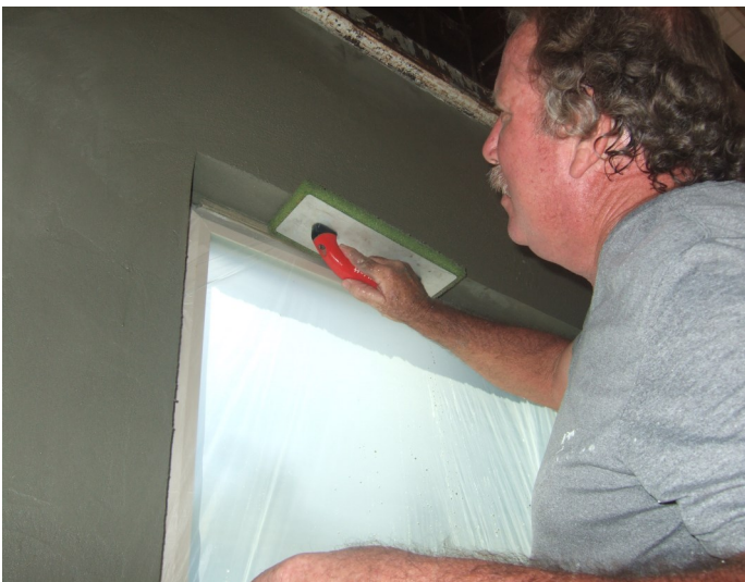
Figure 8-11 Floating the Arris and Window Returns. These are to remain floated and then coated with Drylok. No texture, spray or other finishes that impede water drainage permitted.
